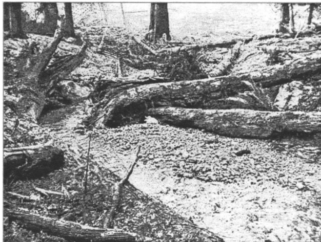
Figure 4. Hannah Creek, December 1999, shows creek reconstruction with logs, jute, and gravel placed to restore fish habitat.
